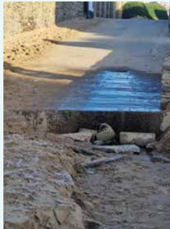
Above: poorly maintained beach access with damaged matting and uneven terrain.
